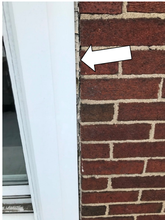
Asbestos Window Sealant
