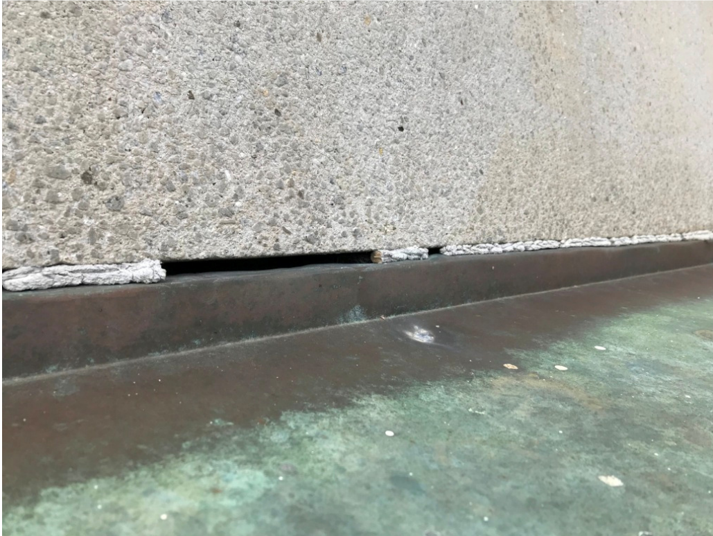
Asbestos White Caulk – North Building East Side Window “Eyebrows”
