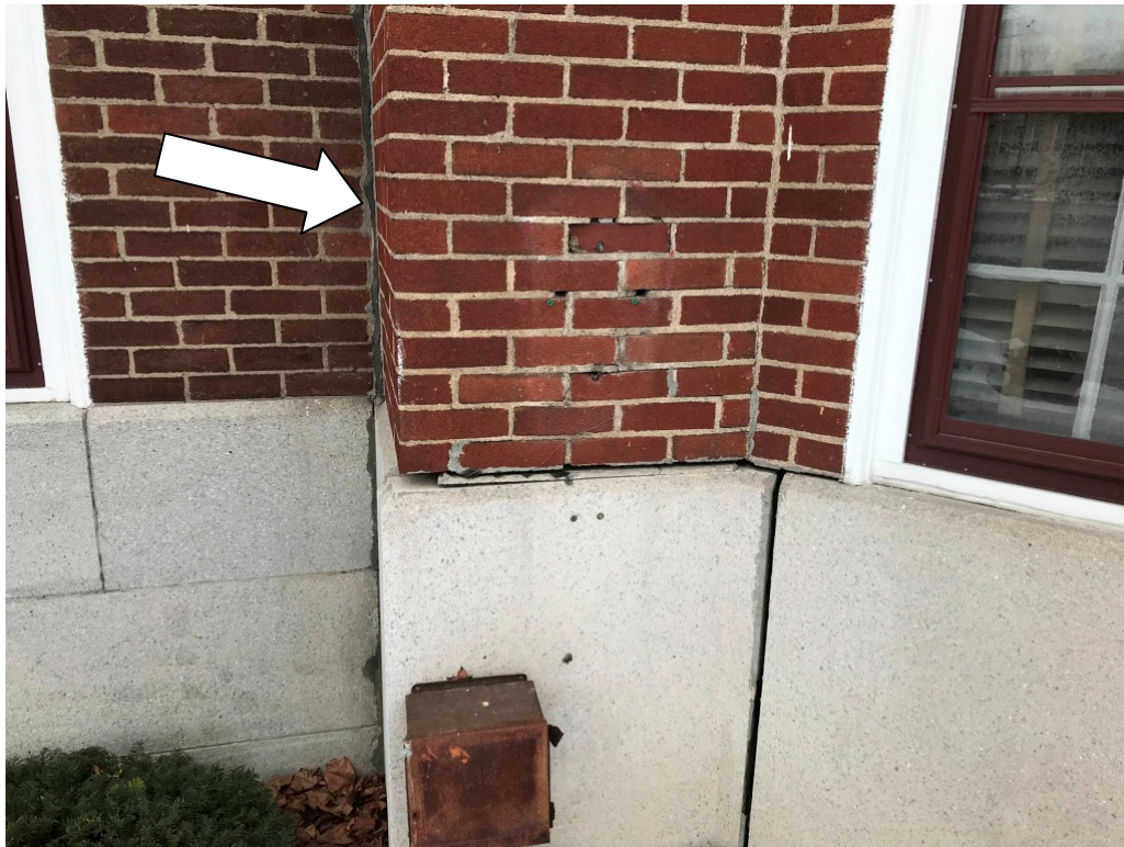
Asbestos Black Tar – North Building North Side Bump Out
