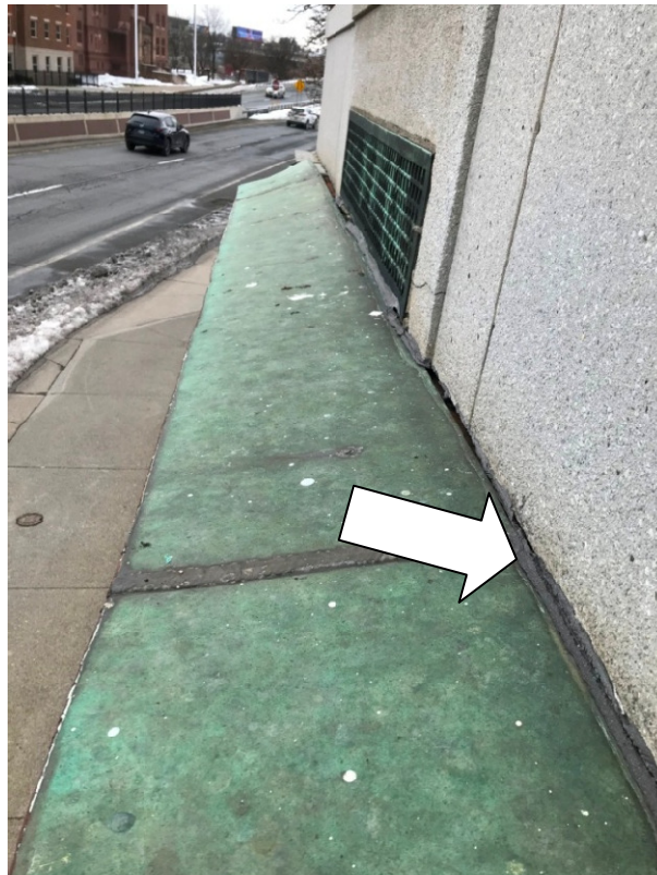
Asbestos Black Tar on Window "Eyebrows" – South Building East Side
