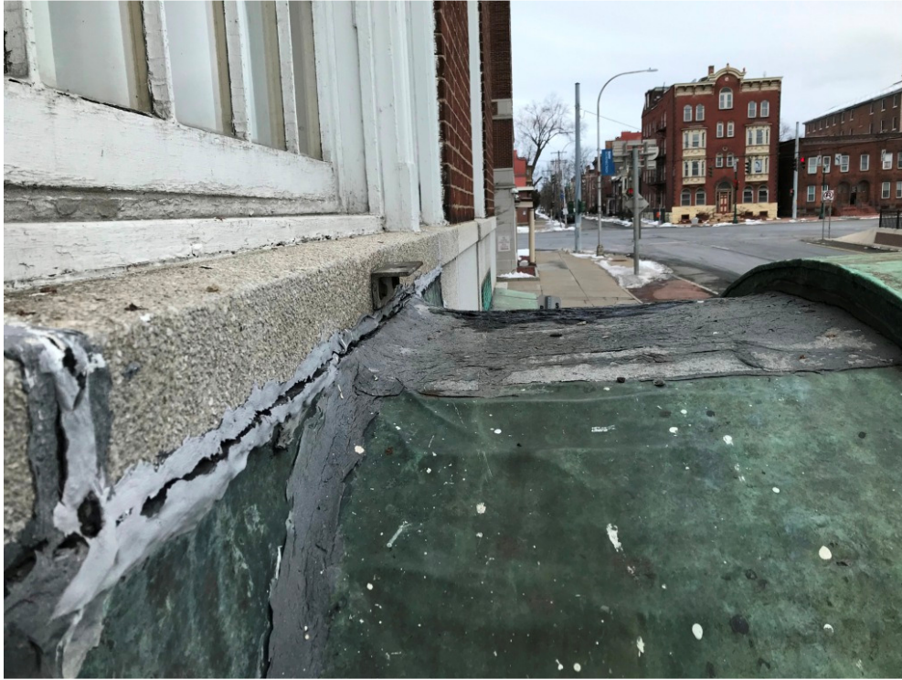
Asbestos Black & Gray Tar on Copper Roof – South Building East Side
