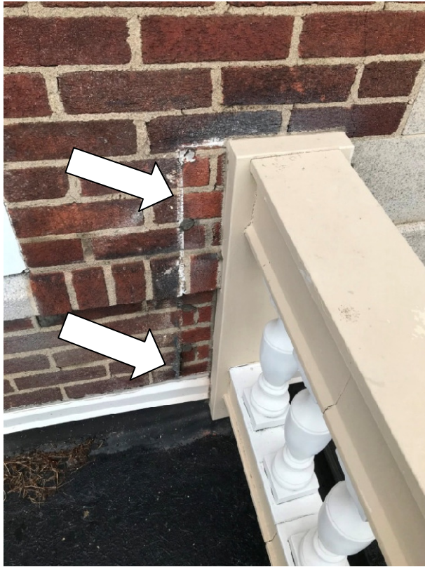
Asbestos Black and White Caulk – Center Core East Side at Old Railing Spot
