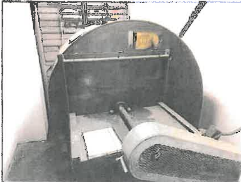
Photo 46: Penthouse exhaust system
