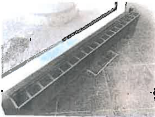
Lobby baseboard heat
