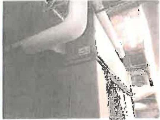
Ninth floor Trane HVAC unit
