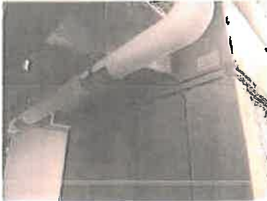
Ninth floor Trane HVAC unit
