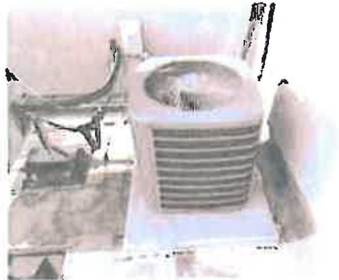
Roof top condenser
